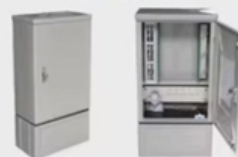
Optical Cable Cross Connection
