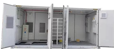
1075KW HH ESS
