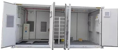
1075KW HH ESS
