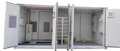
1075KW HH ESS
