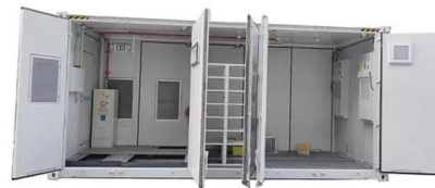
1075KW HH ESS
