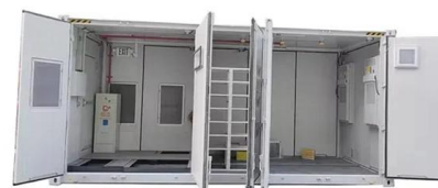
1075KW HH ESS
