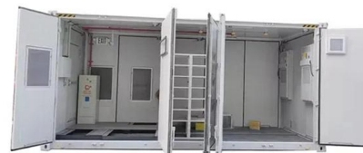
1075KW HH ESS
